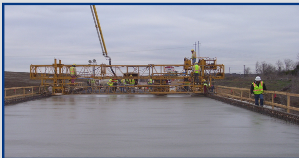
Concrete Deck Placement, SH 130 Southbound Frontage Road over North Fork Dry Creek
