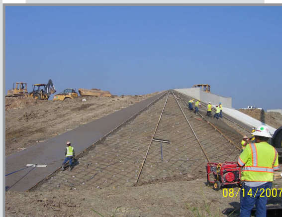
Riprap Work at the McAngus Road Bridge Segment 4 (SH 130 between SH 71 and US 183 South)
