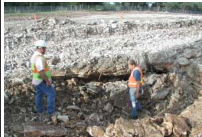
Project field staff evaluate the initial collapse of Outcrop Cave (above).
